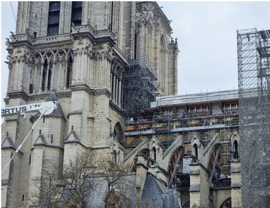
Restoration and reconstruction work at the Cathedral of Notre Dame <Image Source: LEE, Sungyeong>
